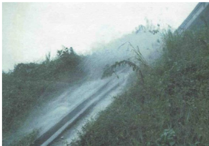
Figure 4: Concentrated flow of surface water commonly due to lack of slope maintenance or deficient drainage provisions
