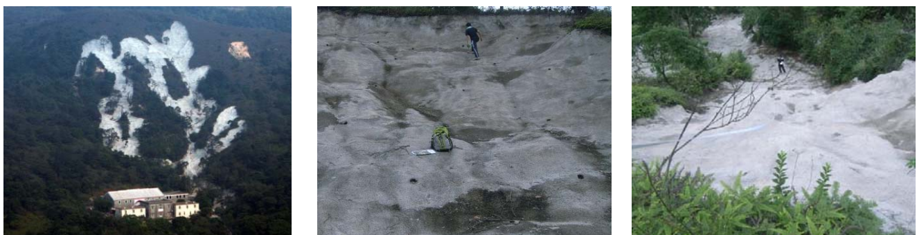
(a) General view (b) Landslide scar (c) Landslide trail Fig. 23. Shotcreting works on the landslide scar in Upper Keung Shan
