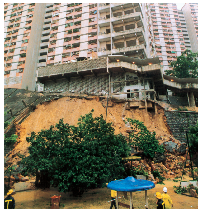
↑ 觀龍樓 D 座對下砌石牆及斜坡塌下，部分地基外露。(The masonry wall and a slope below Block D of the Kwun Lung Lau building collapsed, exposing part of the foundation.)
