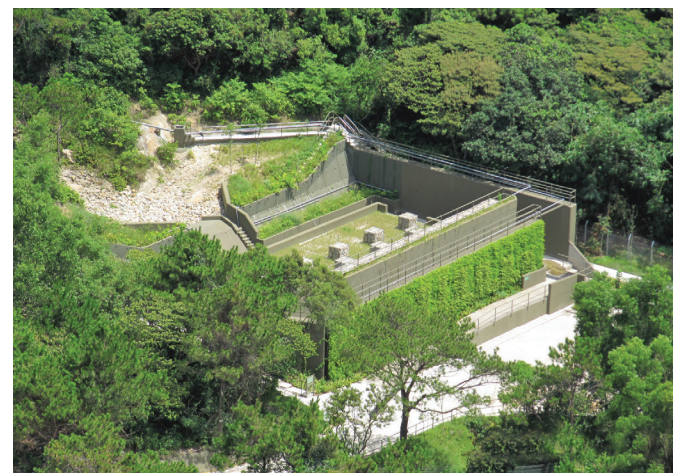
↑ 泥石壩 (Rigid barrier)
