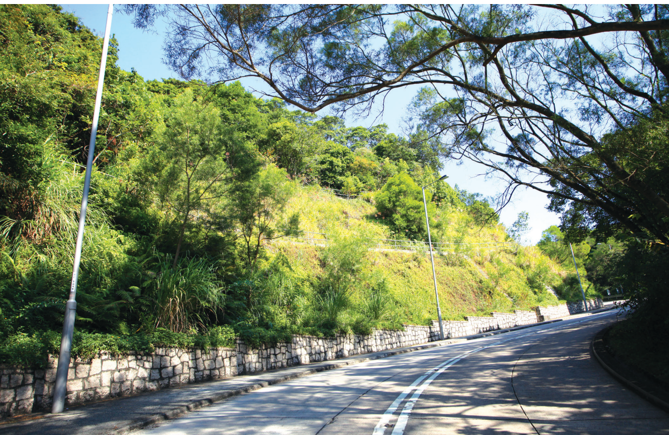
↓ 在斜坡鞏固工程中加入綠化元素 (Greening measures in slope upgrading works.)
