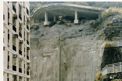
圖6. 樓宇及道路設施非常接近斜坡。 Figure 6. Buildings and roads are constructed close to steep slopes.
