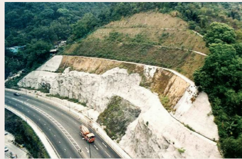
圖5. 建設道路網時亦需切割山坡。 Figure 5. Cut slopes are formed for highway network.
